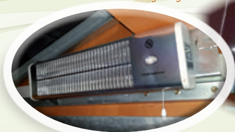
2 chauffages infra-rouge 1200 W. 2 infrared heaters 1200W.
